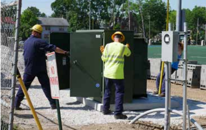
New electrical service
